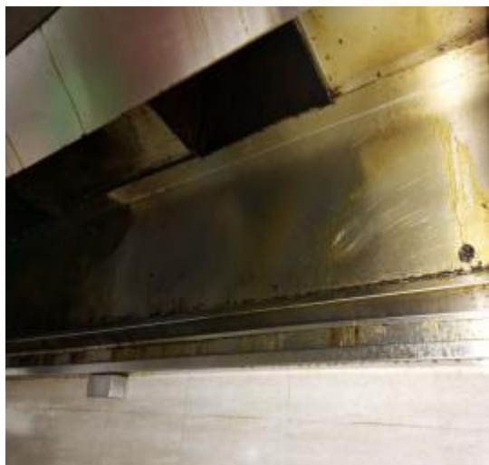
烧腊房烟罩清洗前
