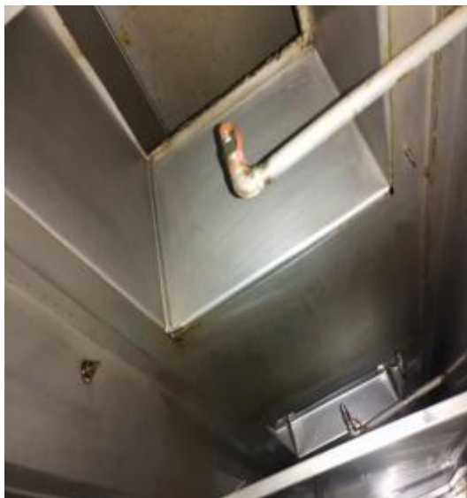
烧腊房烟罩清洗前 1
