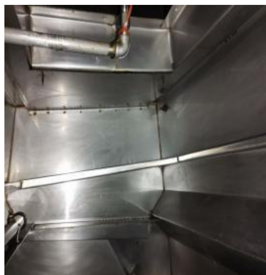
烧腊房烟罩清洗后 1
