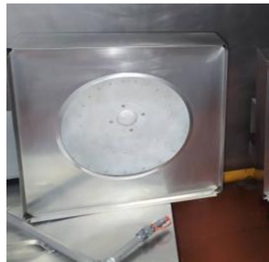
烧腊厨房风轮清洗后
