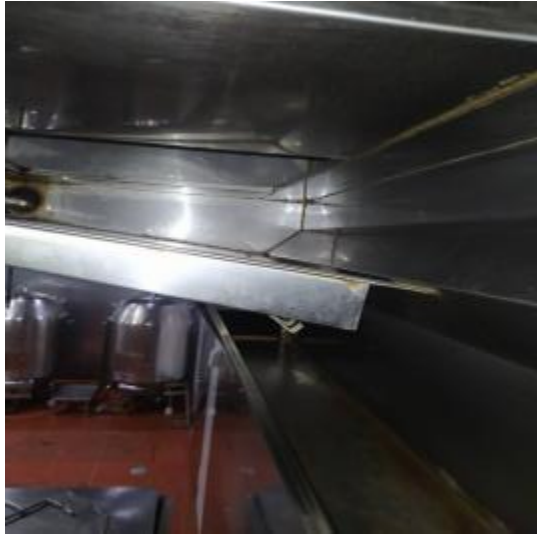
烧腊房烟罩清洗前
