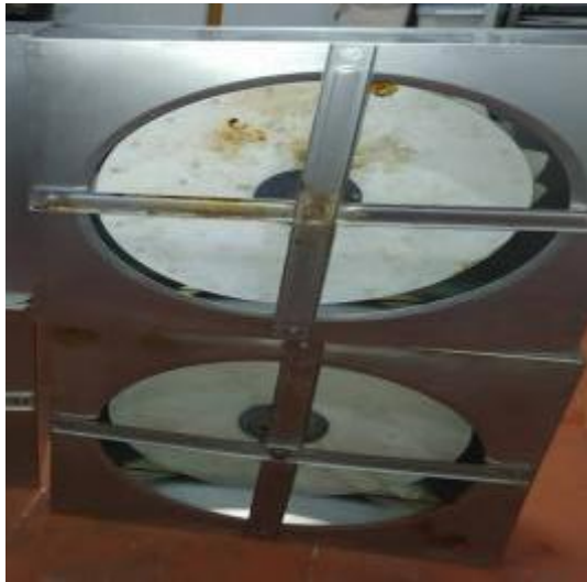
烧腊厨房风轮清洗前
