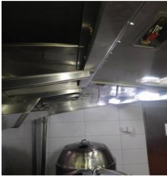
烧腊房烟罩清洗前
