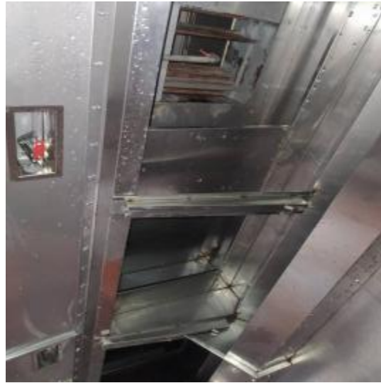
烧腊房烟罩清洗后
