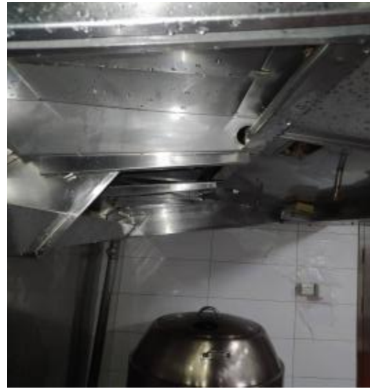
烧腊房烟罩清洗后
