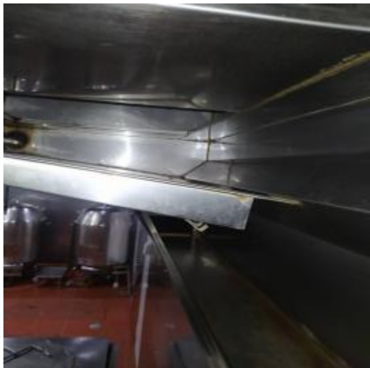
烧腊房烟罩清洗前
