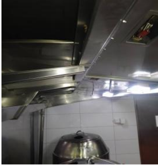
烧腊房烟罩清洗前
