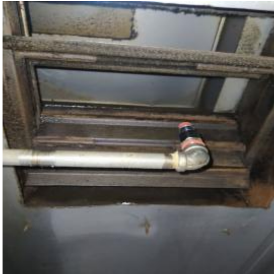
烧腊房烟罩清洗前 1
