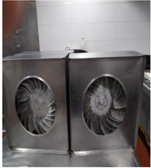
烧腊厨房风轮清洗后
