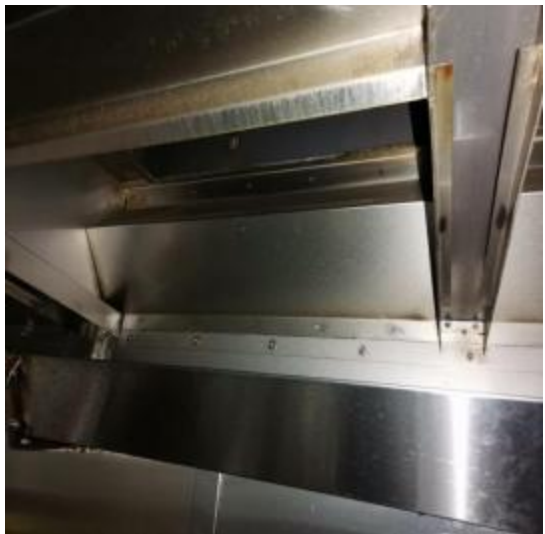
烧腊房烟罩清洗前
