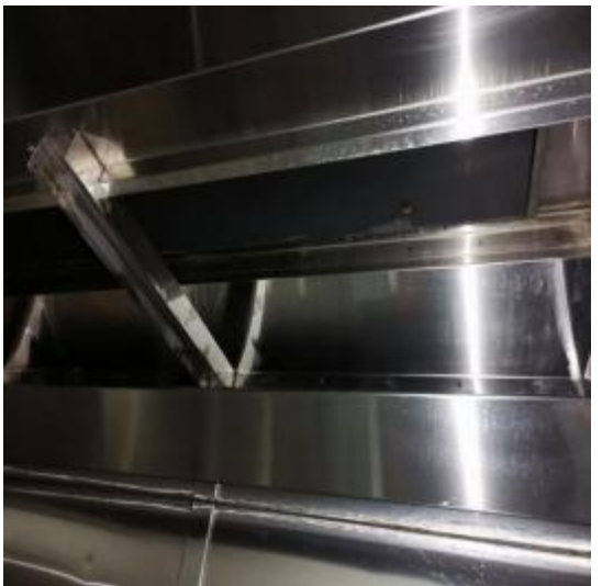
烧腊房烟罩清洗后
