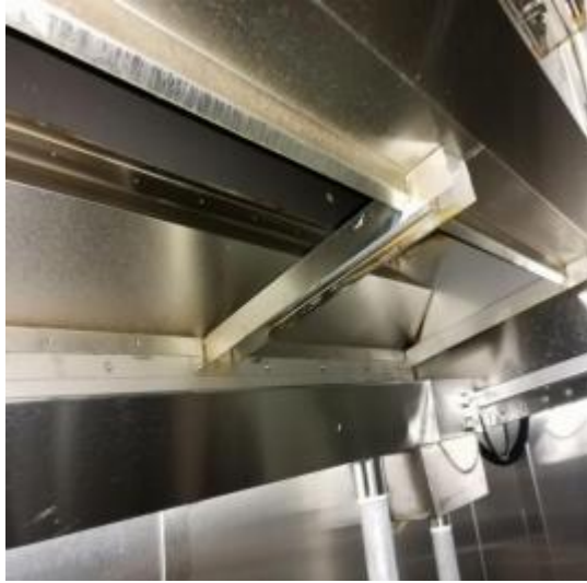
烧腊房烟罩清洗前
