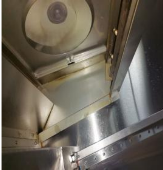
烧腊房烟罩清洗前
