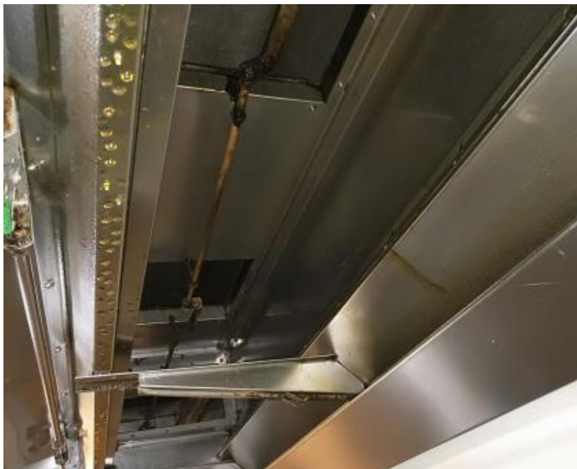
烧腊间烟罩清洗前
