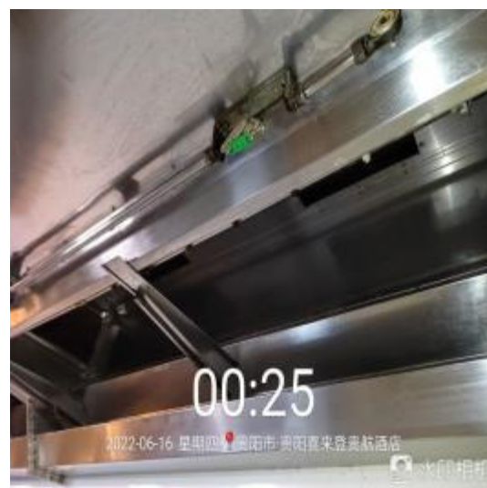
烧腊房烟罩清洗后
