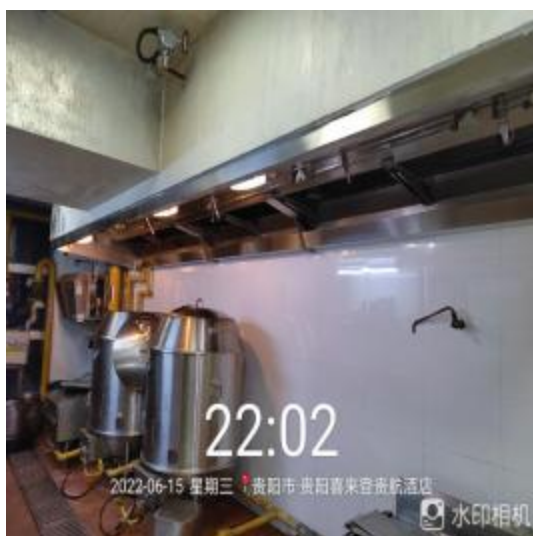
烧腊房烟罩清洗前
