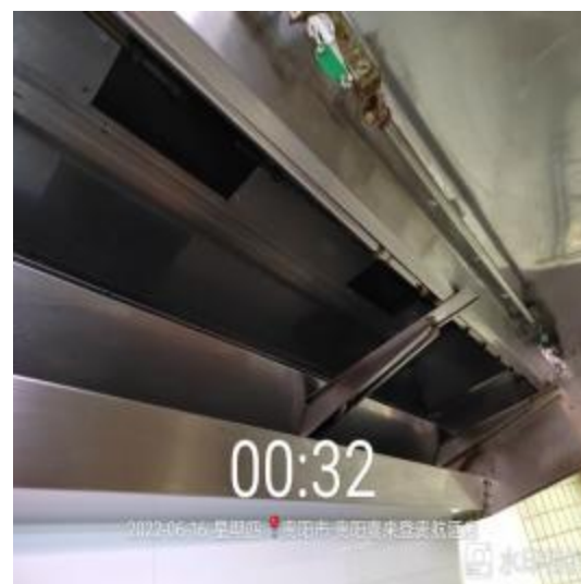
烧腊房烟罩清洗后
