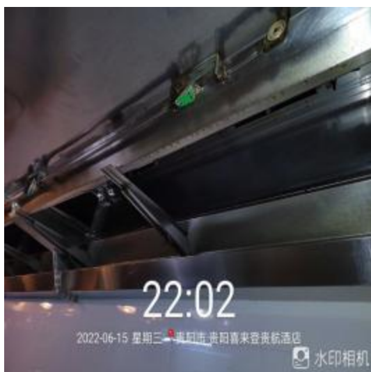
烧腊房烟罩清洗前
