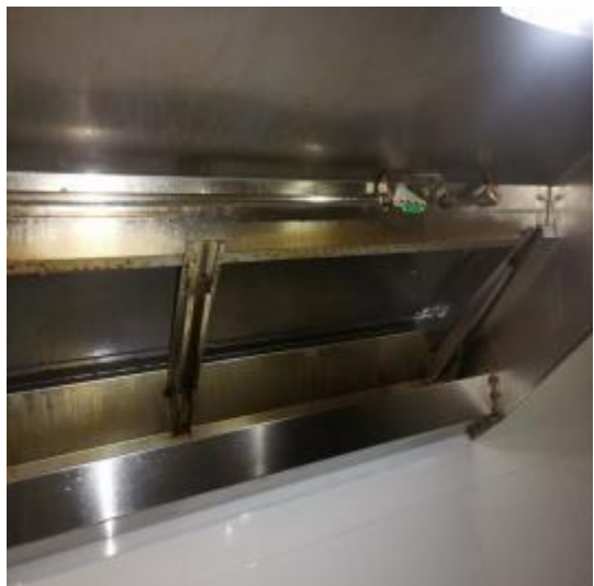
烧腊房烟罩清洗前
