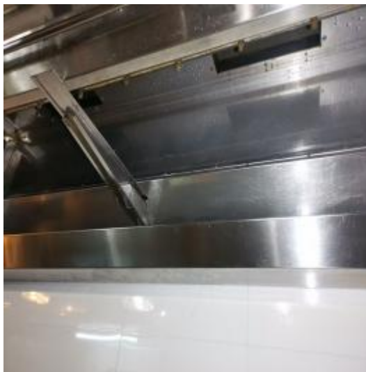
烧腊房烟罩清洗后
