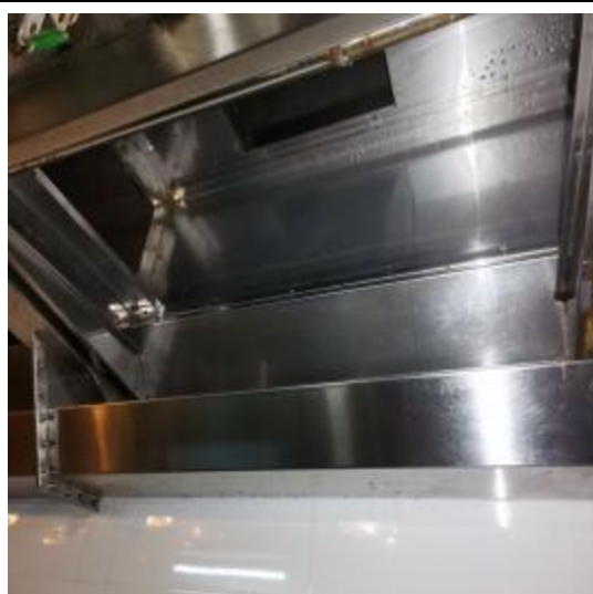
烧腊房烟罩清洗后
