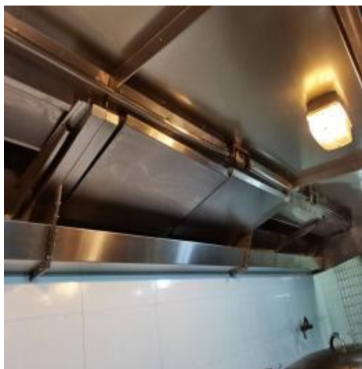
烧腊房烟罩清洗前
