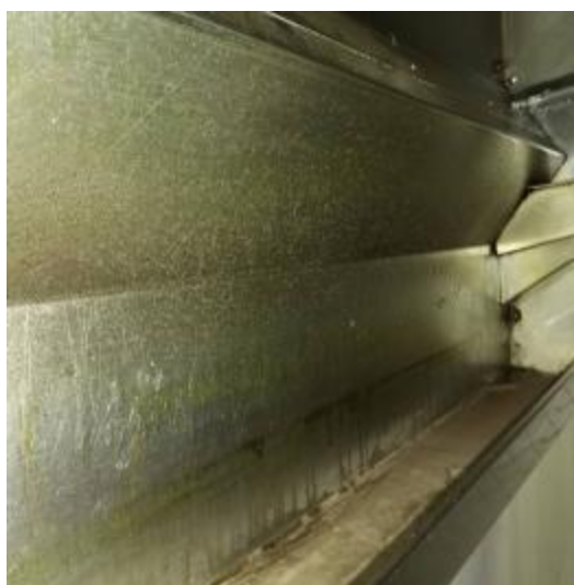
烧腊房烟罩清洗前
