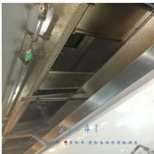
烧腊房烟罩清洗前
