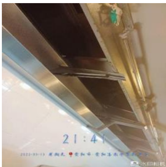
烧腊房烟罩清洗前
