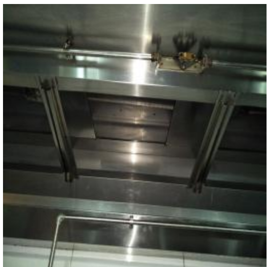
烧腊房烟罩清洗后
