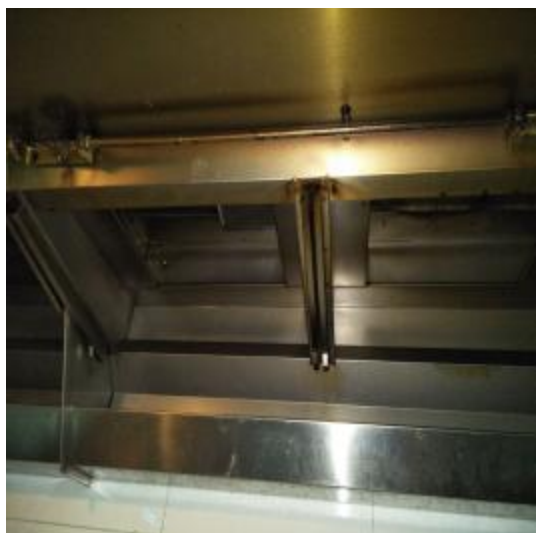
烧腊房烟罩清洗前
