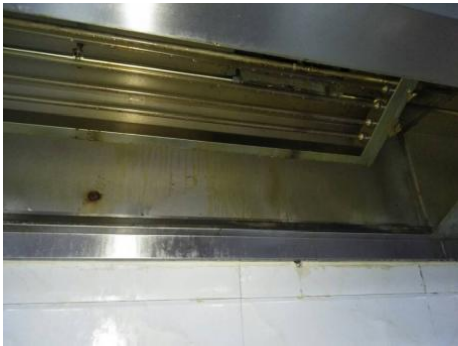
烧腊间烟罩清洗前
